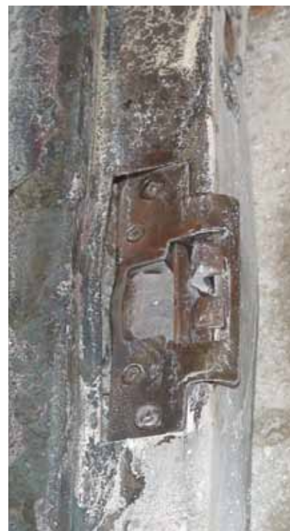
13. View after the test
