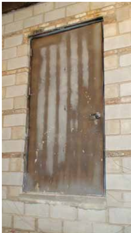
9. Results after heat applied
